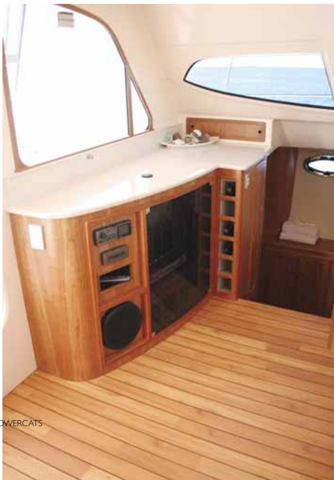
Hard to get enthused over an AC/DC switch panel, but this one was an absolute work of art! (right)
